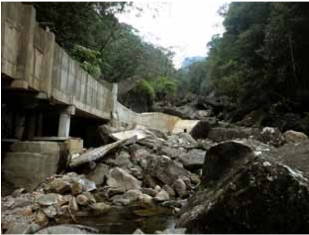
Figure 6. Hydroelectric power plant (note: concrete wall built across the stream and concrete particles dump into the stream).
